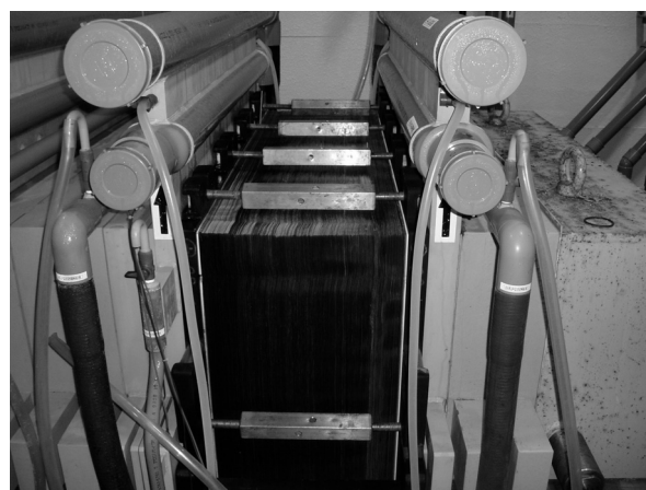
(b)電透析離子交換薄膜清洗槽
