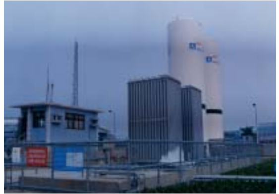
澄清湖淨水場新設液態氧氣槽LOX Tank
