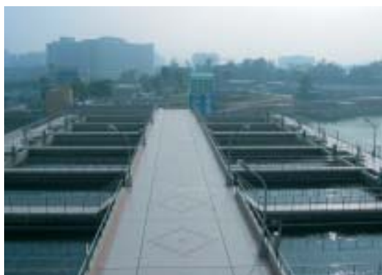
澄清湖淨水場新設快濾池 Mediazor V Rapid Filter
