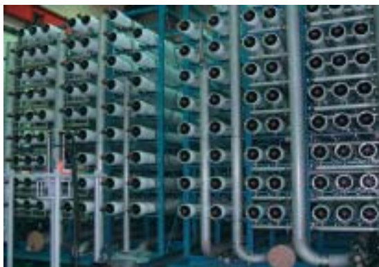
翁公園淨水場低壓逆滲透薄膜 Low Pressure Reverse Osmosis(LPRO)
