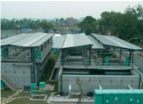
翁公園淨水場超微細浮除設備 Super-fine bubble Flotation Facility
