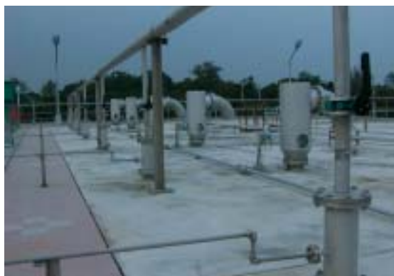
澄清湖淨水場前臭氧接觸池Pre-Ozone Contactor
