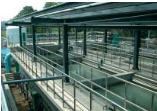
拷潭淨水場超微細浮除設備 Super-fine bubble Flotation Facility
