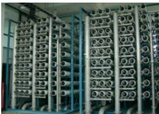
拷潭淨水場低壓逆滲透薄膜 Low Pressure Reverse Osmosis(LPRO)
